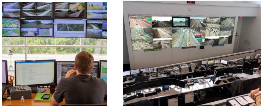
Figure 1-9. VTTI's Smart Roads control room (left) and Transurban's TOC (right).
