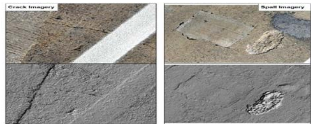
Figure 1: High-resolution 3DOBS output of cracks and spalls
