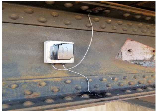
Figure 3: Civionics Wireless Sensor Node on TTCI bridge
