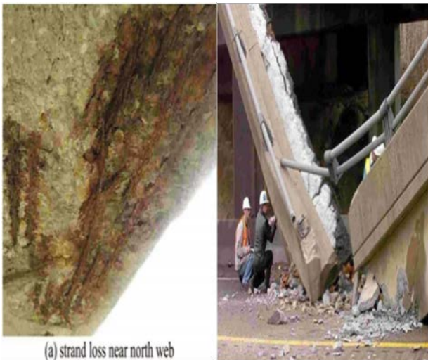
Figure 1: Failures of highways bridges (a) Corrosion of the bridge (b) Collapsed I-70 Lake View Drive Bridge, Pittsburgh, PA
