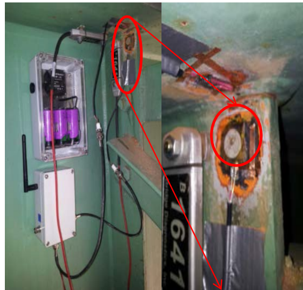
Figure 1: Wireless AE Sensor (Left) and Crack (Right)
