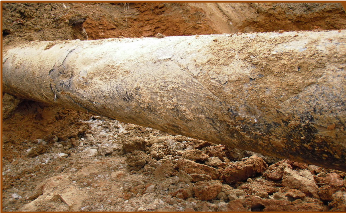
While a car can survive a dent and flaking paint, a pipeline with a dent of this significance (see left side) and deteriorating coating, requires immediate repair or replacement.
