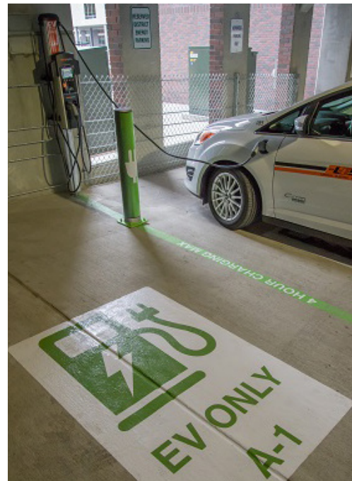
Current LES Charging Stations in Lincoln
