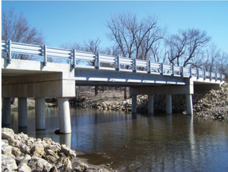
Figure 7 Ultra-high performance concrete pi-girders were used in the construction of the Jakway Park Bridge in Buchanan County, Iowa.
