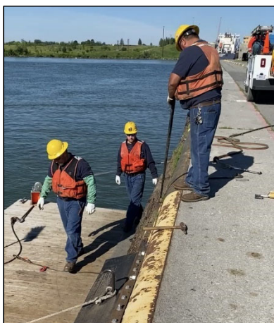
GLS work crews perform fendering replacement along the lower guidewall at Eisenhower Lock.
