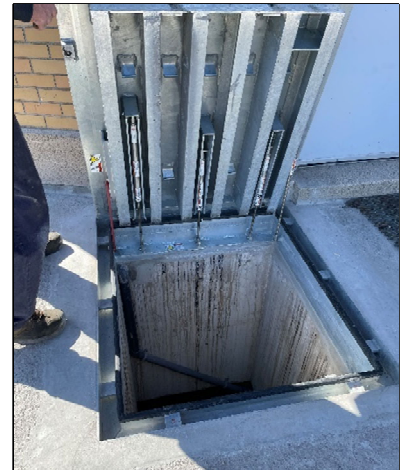
An example of one of the new personnel access hatches along the lock wall to keep water out of recesses and provide improved safety for GLS personnel.
