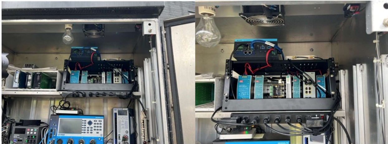
Figure 23 Left. In large signal control cabinets, the space allows all additional sensing equipment to be co-located with the signal controller. Right. Zoom in on the lidar installation.
