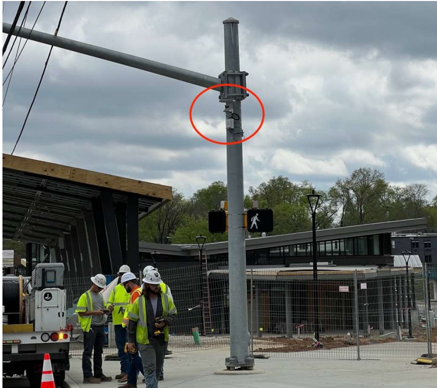
Figure 6 Detail of lidar sensor installation from Stage 1 intersection 26th Ave. And Clarksville Pike. The sensor and its power adapter are circled in red.
