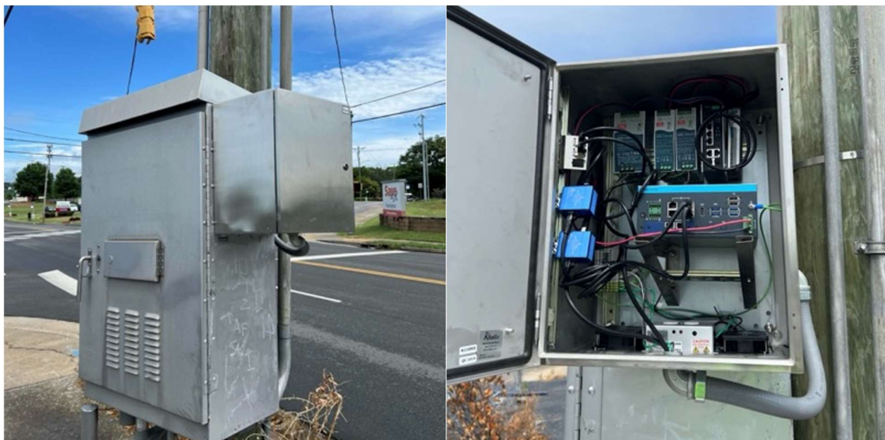
Figure 70 Left. Typical installation includes a small additional cabinet attached to the main signal control cabinet. Right. Cabinet includes the edge computer power supplies, and a network switch.
