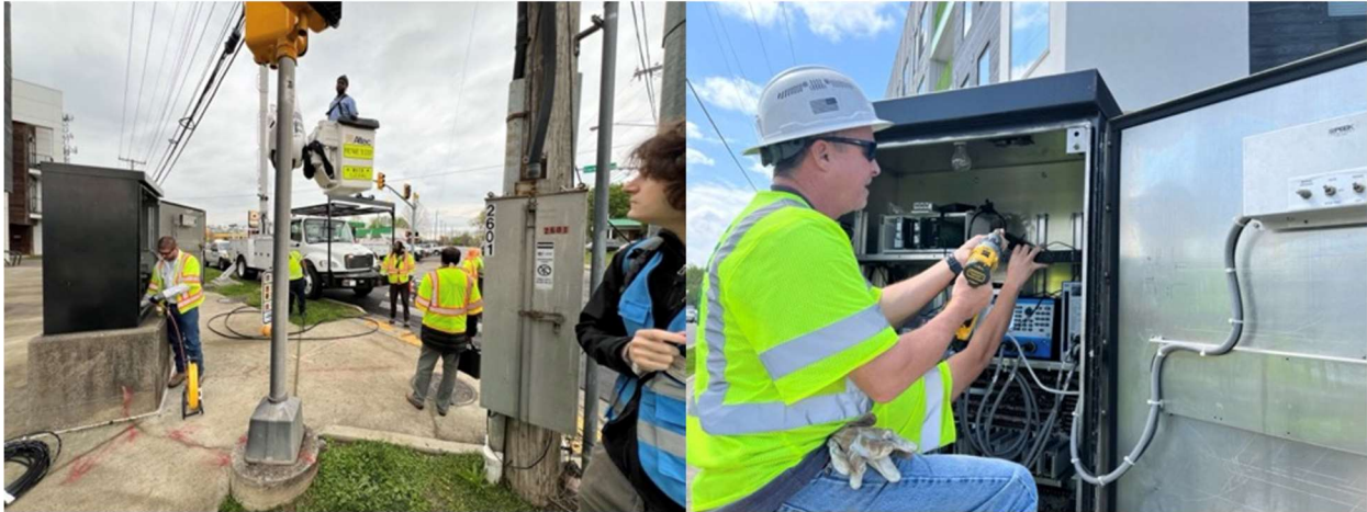
Figure 22 Photos from the first LADDMS lidar installation located at 26 th Ave and Clarksville Ave. in April 2024.
