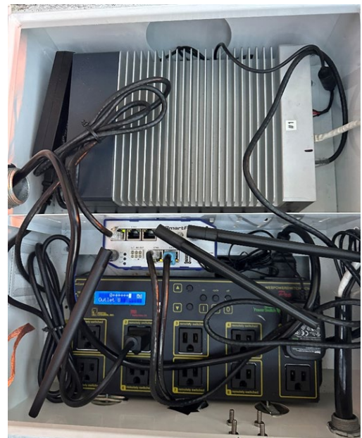
Cabinet assembly: AI Edge Processing and AI Mobile Edge Processing, includes a wireless 4G/5G router, AI edge processor unit, and web-managed power strip.
