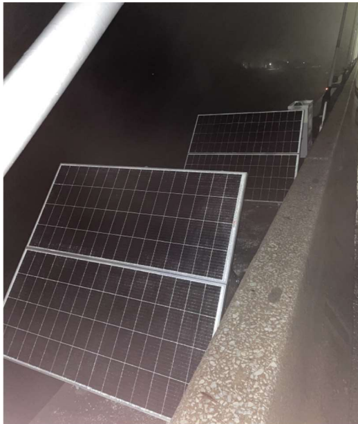
Figure 13 - Solar Panels Attached to the Bridge
