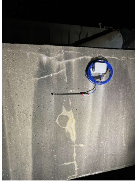
Figure 8 – Crackmeter Placed at Existing Crack
