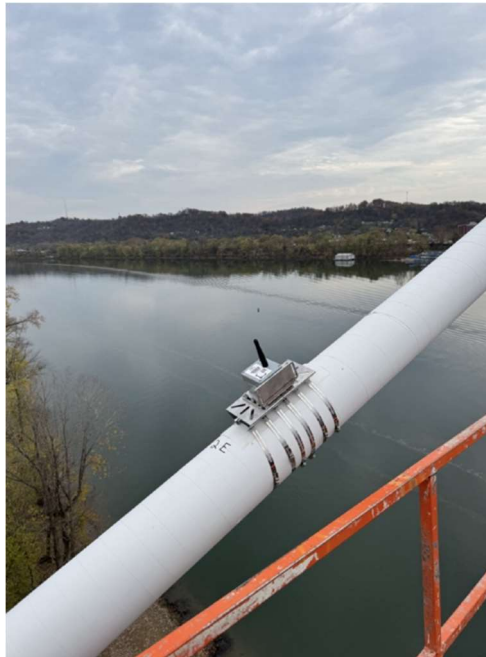
Figure 3 – Accelerometer Installed on a Stay Cable
