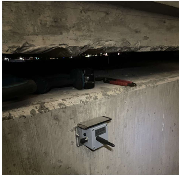
Figure 7 – Vessel Collision Detection Sensor Attached to Concrete
