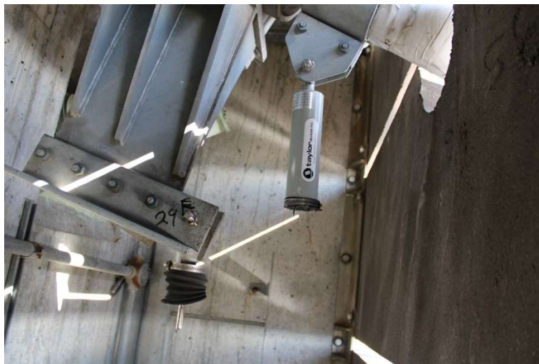
Figure 20 – Photo of Broken Damper at Cable E29
