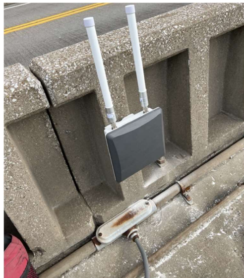
Figure 11 – Gateway Attached to the Bridge
