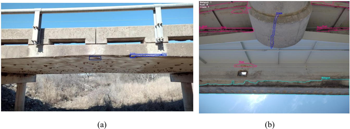
Figure 8. Detection of small defects that are difficult to see on Cowley and Sedgwick County bridges using YOLOv11: (a) Spalling identified on the underside of the bridge deck (Structure No. 000000000180890); (b) Small rust fragments detected on bridge girders (Structure No. 000000000870040).
