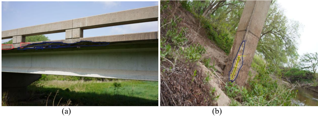
Figure 7. Concrete defect detection on Saline County bridges using YOLOv11: (a) Large spalling area identified (Structure No. 000000000850950); (b) Simultaneous detection of rust, spalling, and exposed rebar at the same location (Structure No. 000000000850770).
