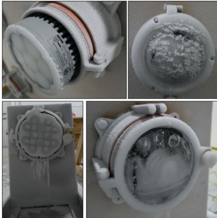
Figure 17. LED light fixtures after 30 minutes of operation at -20 degrees. Source: FRA
