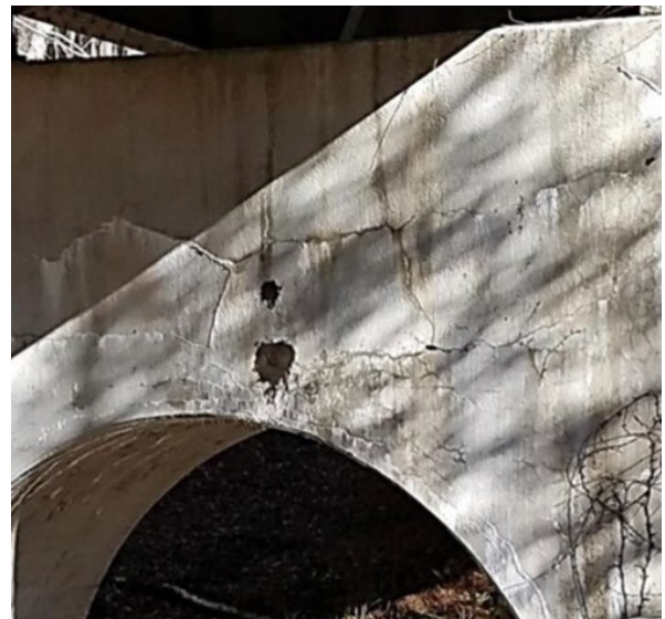
Figure 10. An example of concrete cracking caused by alkali-silica reaction gels. Source: FHWA
