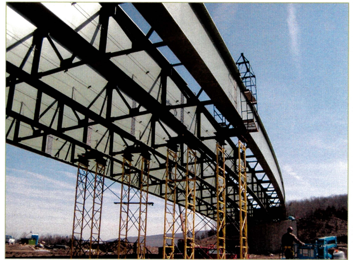
Superstructure of Bridge #207, carrying State Route 322 over Interstate 99 in Centre County, PA, showing shoring (yellow) used to stabilize horizontally curved steel girders during construction. Researchers from Penn State’s Larson Institute are developing better approaches for designing and analyzing curved and skewed structures during construction to ensure that costly and hazardous fabrication mistakes are a thing of the past.
