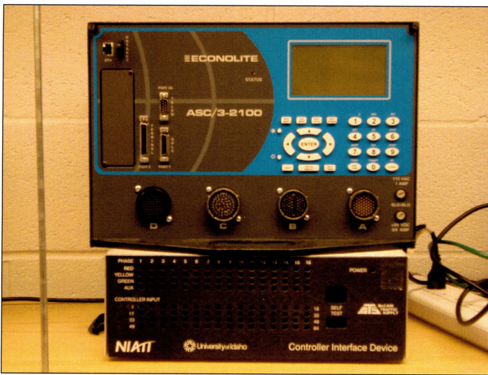
Econolite ASC/3 traffic controller atop NIATT controller interface device (CID)
