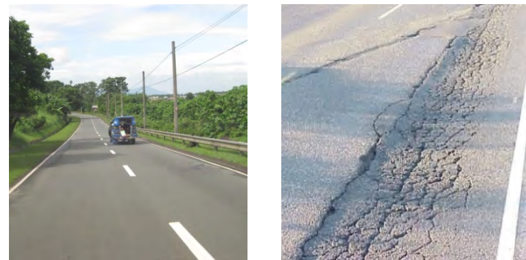
Figure 3.8. Pavement Condition, Good vs. Poor
