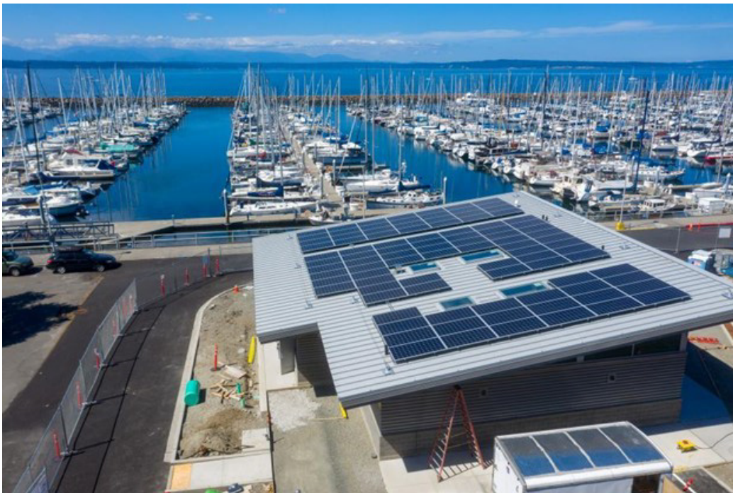
Solar panels at Port of Seattle (Image source: Port of Seattle)
