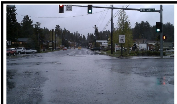
The lack of stormwater facilities in the project area creates flooding during heavy rain or rapid snow melt and compromises water quality.
