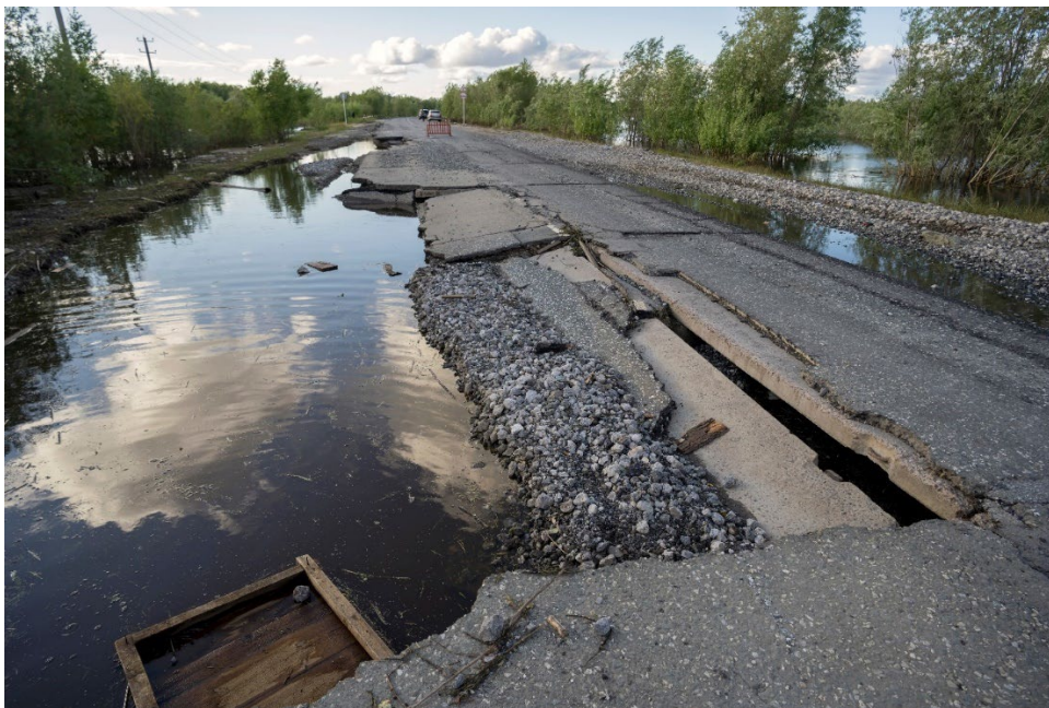
Roadway damaged by flooding
