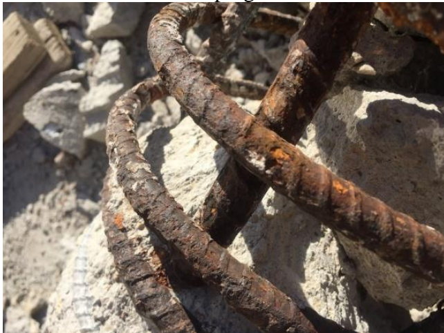
Corrosion-damaged reinforced concrete column
