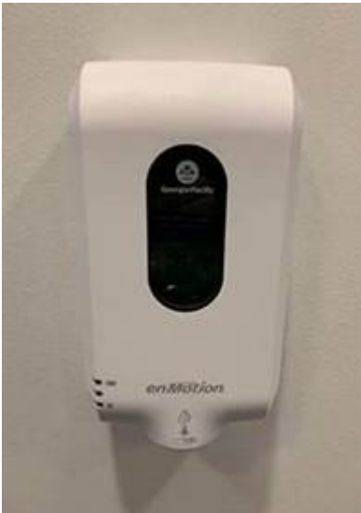
Wall Mounted Hand Sanitizer Stations in all elevator lobbies above the ground floor
