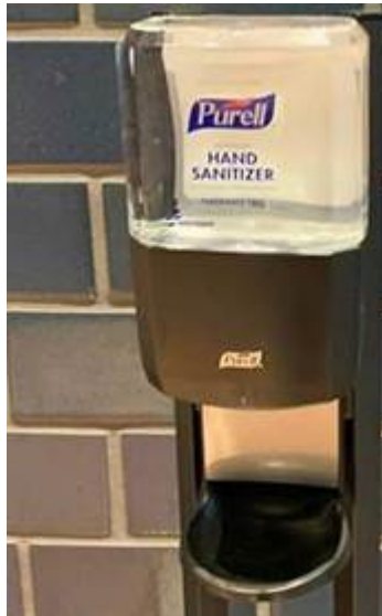
Freestanding Stations in the Shuttle Elevators and Ground Floor Elevator lobbies
