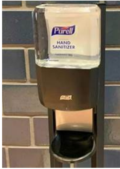
Freestanding Stations in the Shuttle Elevators and Ground Floor Elevator lobbies
