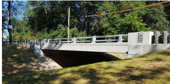
Figure 8. Delaware DOT combined precast elements with UHPC connections and a UHPC overlay on an Accelerated Innovation Deployment Demonstration project.
