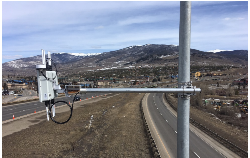
A pilot project C-V2X roadside unit mounted above I-70 along Colorado's Mountain Corridor.
