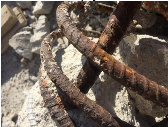
Corrosion-damaged reinforced concrete column
