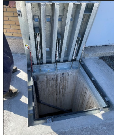
An example of one of the new personnel access hatches along the lock wall to keep water out of recesses and provide improved safety for GLS personnel.
