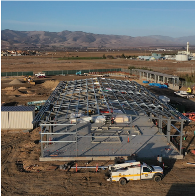
Project underway after Monterey-Salinas Transit District received a TIFIA loan in 2020 for a rural bus facility.
